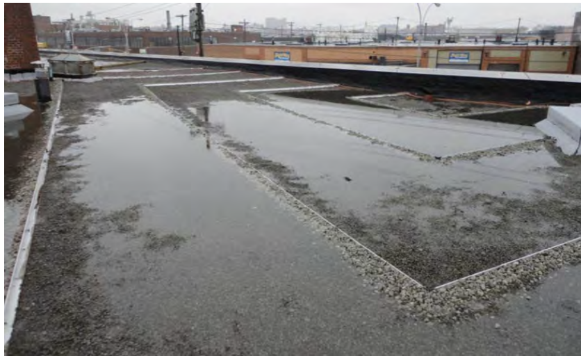
FIGURE 7-3 BLUE ROOF SYSTEM UTILIZING CHECK DAMS TO RETAIN STORM WATER SOURCE: GEOSYNTHETIC CONSULTANTS
