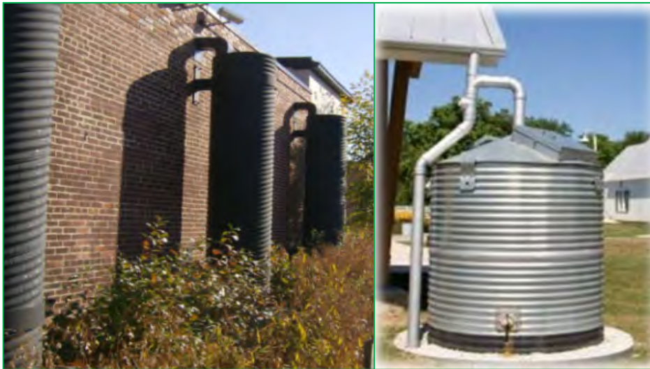
FIGURE 7-2 TYPICAL ABOVE-GROUND RAINWATER HARVESTING CISTERNS
